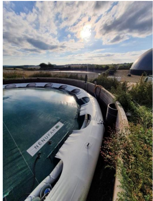
Image 5. External pit equipped with a cover for passive anaerobic digestion.
